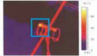
Component: 220kv connector isolator Defect type: heat due to poor connection at ring gag connector
