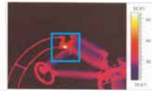
Component: 500kv breaker connector Defect type: breaker connector heat
